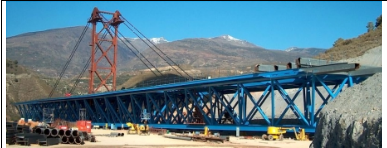
Figure 6 General view during erection of the steel truss on the access to the South abutment
