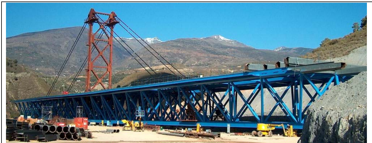
Figure 3: General view during erection of the steel truss on the access to the South abutment
