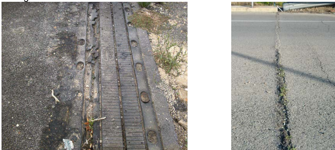
Figure 6 – Damaged expansion joint . Non existing expansion joint
