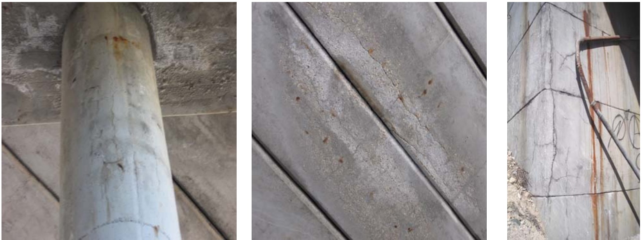
Figure 2 – Some crack son piers, decks and front walls
