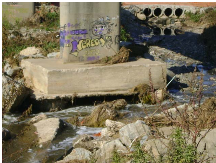
Figure 3 – Scour effect on the foundation of a pier
