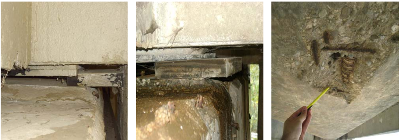
Figure 11 – An elastomeric bearing out of place, and a lack of cover of a prestressed tendon.
