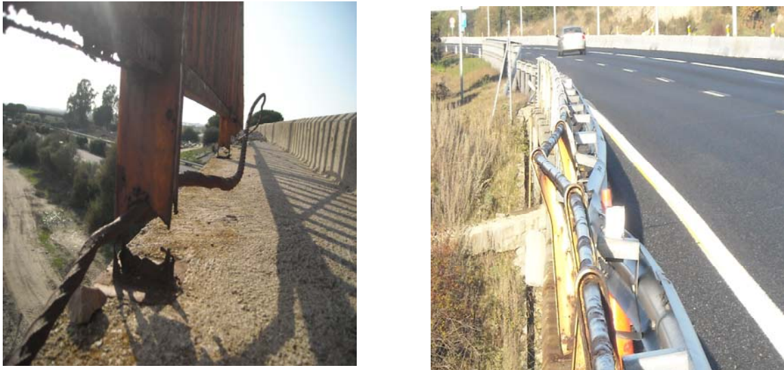
Figure 7 – Damages on steel guardrails and barriers
