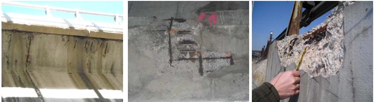
Figure 4 – Loss of the cover and corroded reinforcing. Spalling of the concrete.
