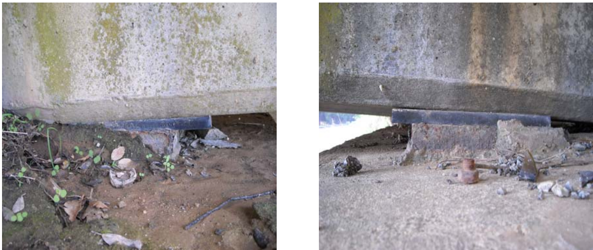
Figure 5 – Blocked bearings o out of place
