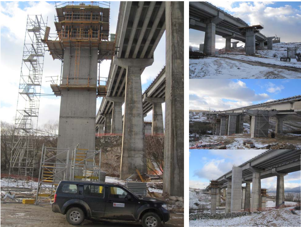
Figure 12 – General views of the repairing works of some bridges of the AP-6
